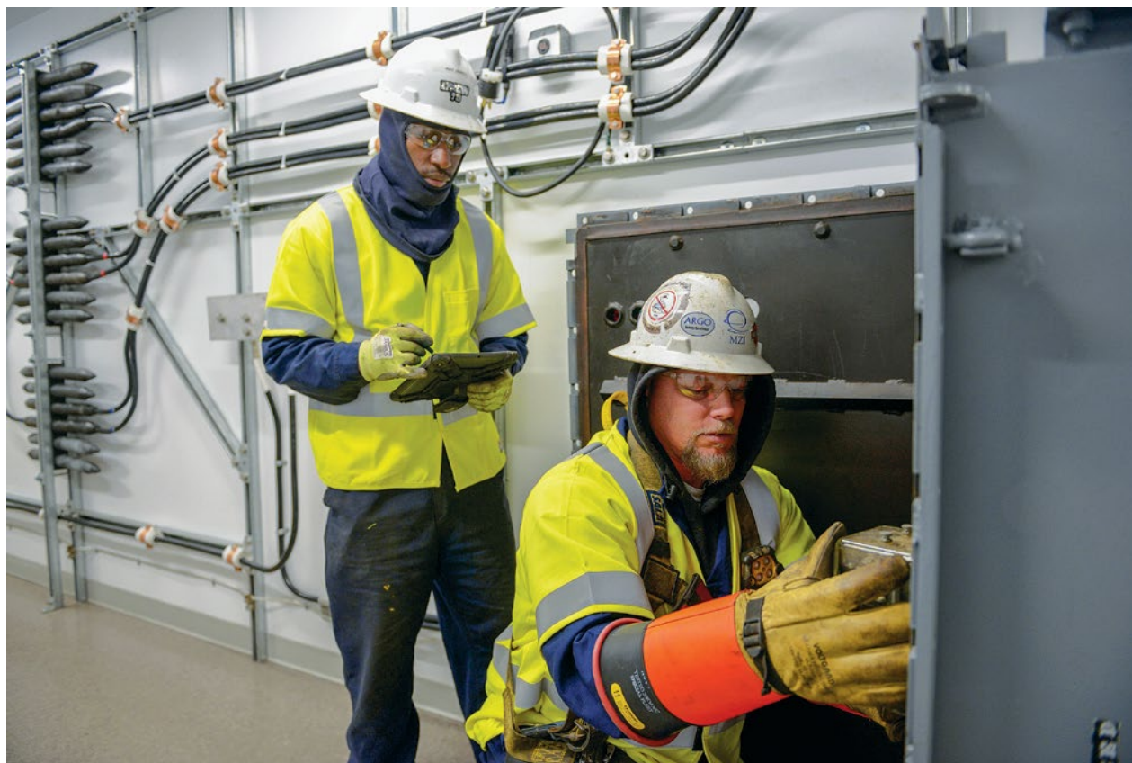
Clockwise from top: Turray James and Andy Chomor assess conditions on a network protector; Aldridge project engineer Chet Chippie with general foreman John Ficetti; and the Aldridge safety trailer, a converted race car hauler with a simulated manhole cut into the top.
